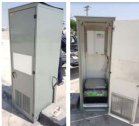
Fig.7 – Outdoor test for an SMC battery, high temperature environment
