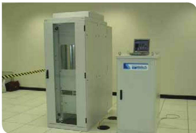
Fig. 5 Idatech 3kW Fuel Cell installation with a 3kVA Chloride UPS
