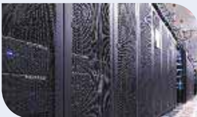
Protection of small-medium size servers - all sectors
