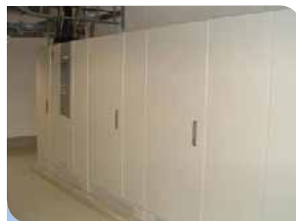
800 kVA 90-NET UPS systems
