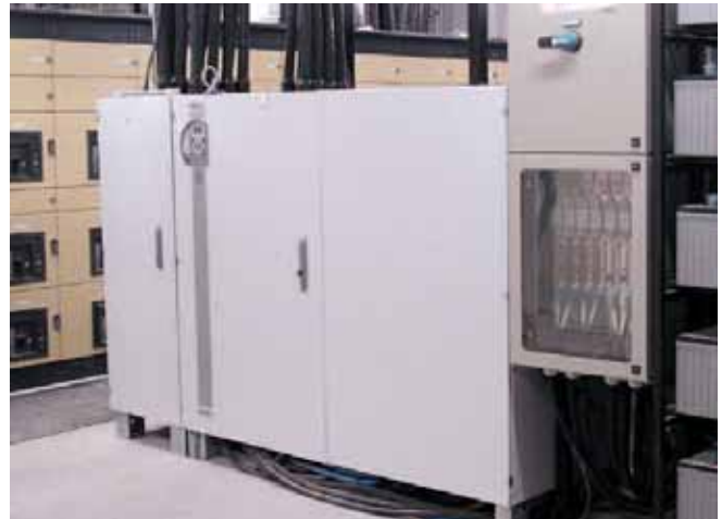
Chloride 90-NET 500 kVA UPS installation
