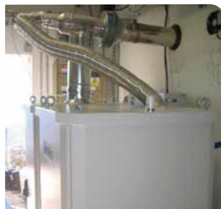
Fuel Cell systems and reformer module
