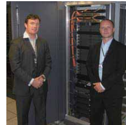
Andrew Clarke and William Barrell, Infrastructure Project manager, pictured with Chloride's Active UPS. Deployed across ten communications rooms to support the IPT deployment, Chloride's Active 3000VA is installed in standard cabinets with MODBUS and SNMP cards, to ensure that voice communications are not lost in the event of power failures. Testing showed that the Chloride batteries will support the system at full load for 30% longer than the designed specification.
