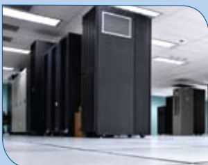
Small to medium datacenters
