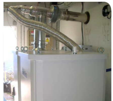
Fuel Cell systems and reformer modules
