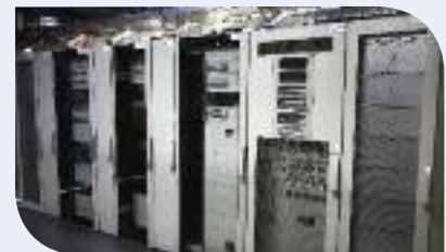
Protection of large data centers - all sectors
